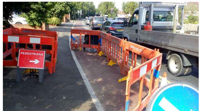
Whilst this worksite has space available to pass, the layout pushes people walking and cycling together.
