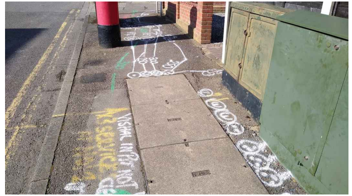
The hidden tangle of buried cables and ducts marked out before repair works.
