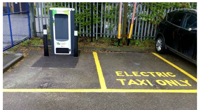
Rapid charger in a car park for taxis.
