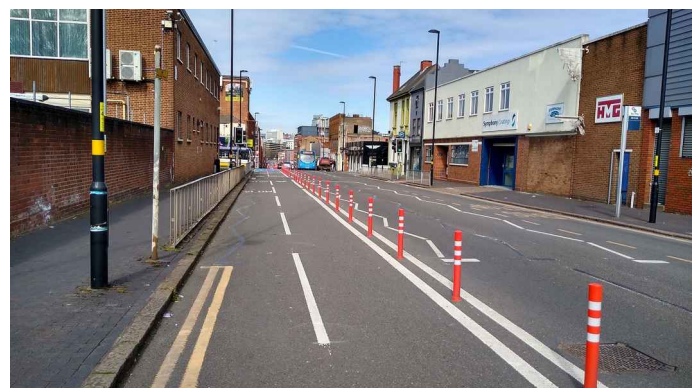
Bradford Street, Birmingham. An experimental reallocation of road space allowing the live testing and evaluation of a street layout.
