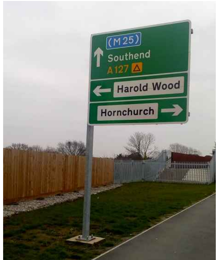
This large trunk road traffic sign has been installed in the verge with a cantilevered frame to avoid a second post placed into the footway.
