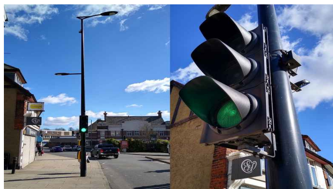
This traffic signal is placed on a lighting column
