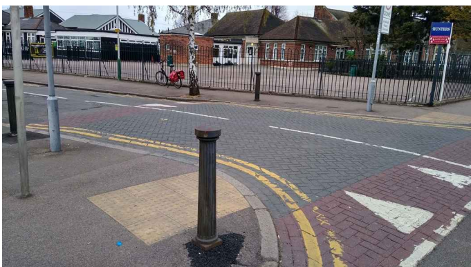
Bollards protecting the crossing points at this side street. The nearest one has been recently reset after being knocked over.
