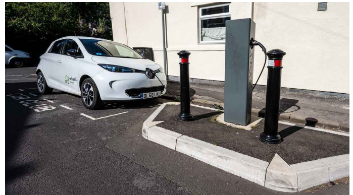
EV charger placed on a carriageway island, Carlyle Road, Bristol.
